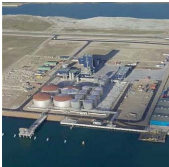
This tank farm is equipped with Pulsair system for inerting plus stirring. The four tanks in the lower left have a content of 14,700 cu m each, filled with biofuel (Fig. 3).
