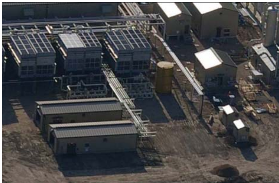
The injection pumps are in the two long buildings in the lower left. The pipe rack coming out of pump buildings goes towards the aerial compressor coolers. Two variable-frequency-drive buildings are to the right of the pump buildings. Two transformers are behind the VFD buildings. The Heat exchangers' open skid is visible behind the pump-skid building (Fig. 1).
