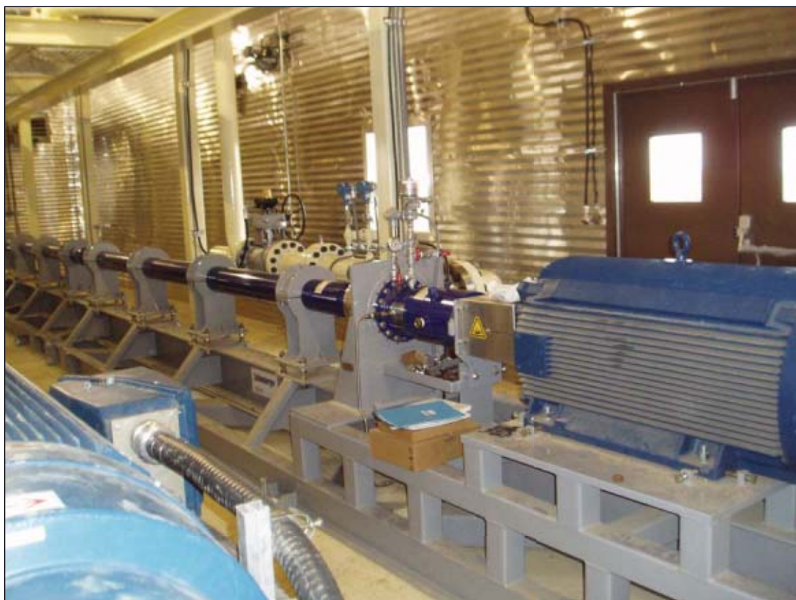
Each injection pump building houses two Reda pump skids (Fig. 2).
