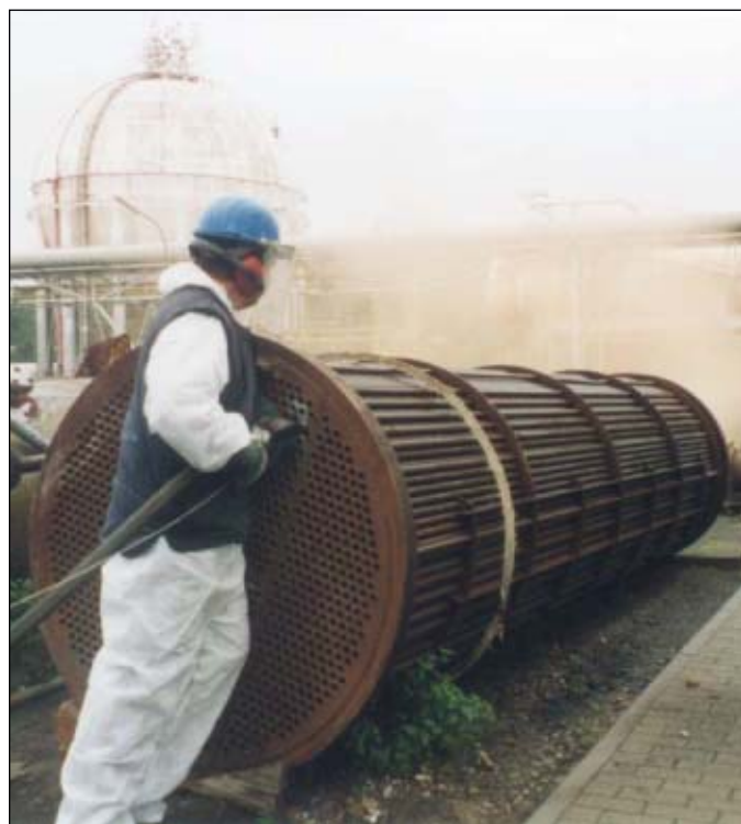
Cleaning pipes in a heat exchanger in the chemical industry uses the CryoClean process (Fig. 8).
