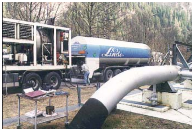
A pig trap and nitrogen injection point was installed for this pipeline restoration at Rongellen, Switzerland (Fig. 7)
